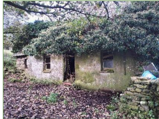
Plate 3.2 Derelict structure (S_03 in Figure 3.3) present east of the proposed Turbine 7 displaying 'low' suitability for roosting bats.
