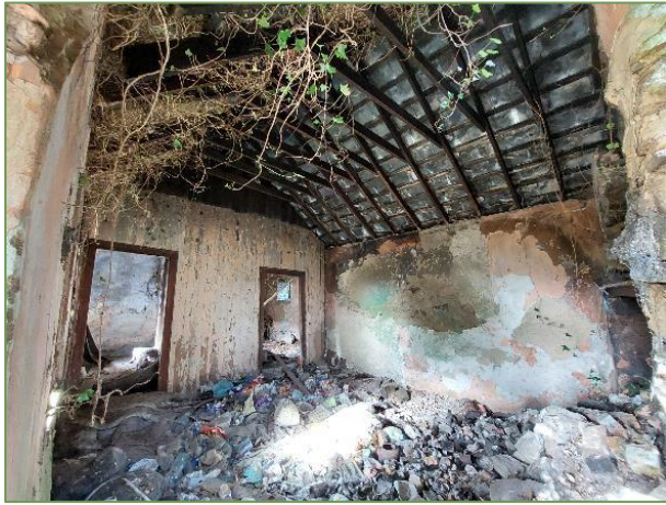
A5. Interior of the derelict structure S_03 . Partial Slate roof remaining with significant light ingress
